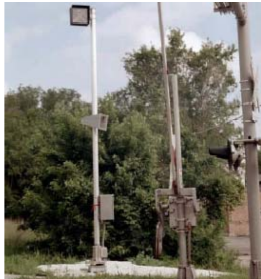
Figure 5. AHS Installation in Mundelein
